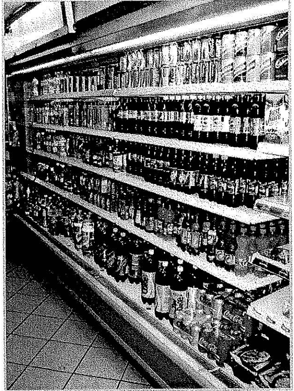
Soft Drinks Chiller Unit
